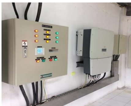
Gambar 3. Inverter PLTS Rooftop on grid kapasitas 30 KVA
