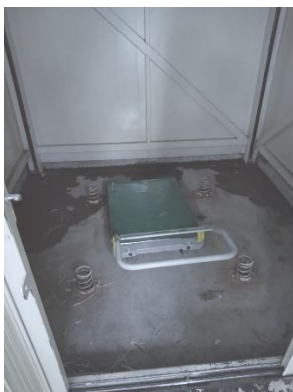
Gambar 1. Trolley terhimpit lift barang
